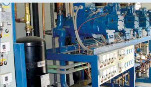
Energy and performance monitoring
